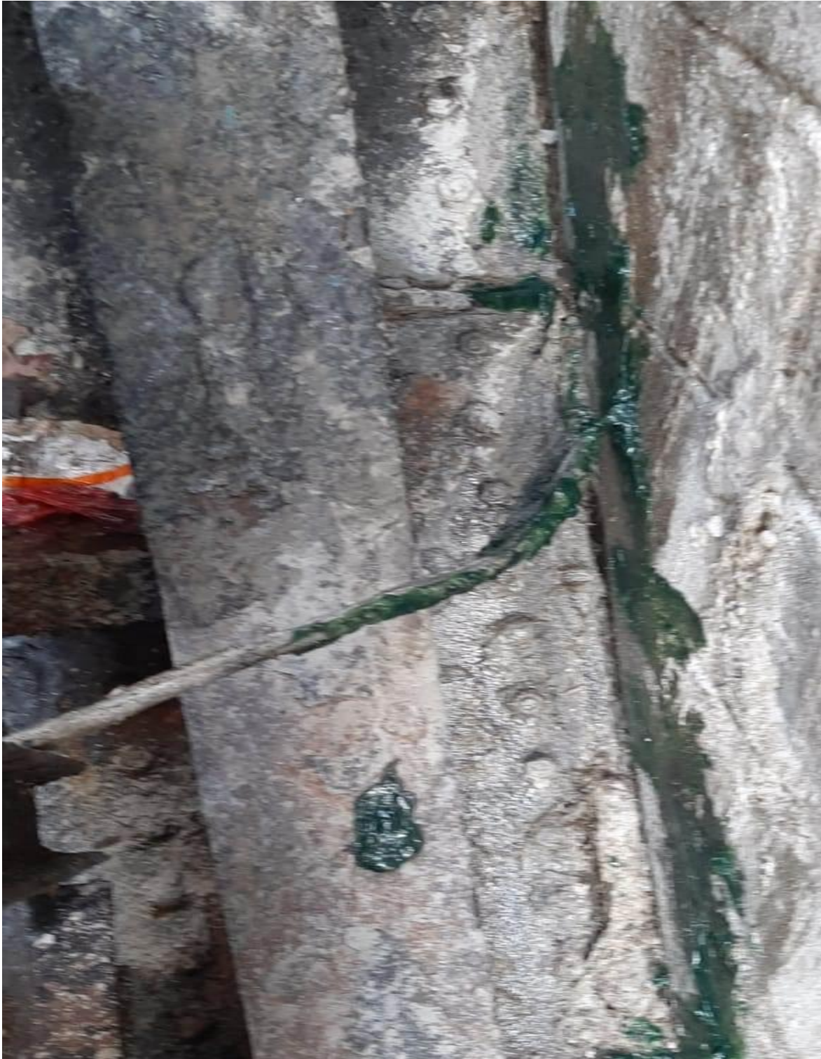
Spillway damaged rubber seal
